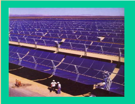
Central Solar Energy
